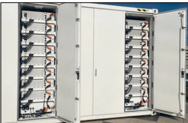
Battery Energy Storage Systems
